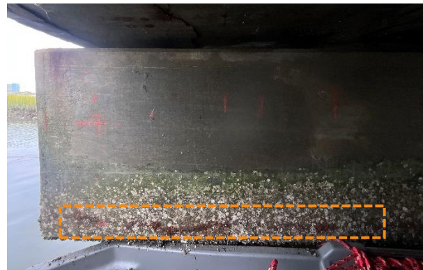
Figure 6. Visible corrosion byproduct and cracking on bottom longitudinal reinforcing layer on bent cap 3.
