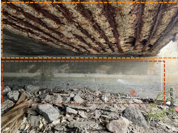
Figure 4. Representative deterioration of existing bridge deck in orange box and good condition of bent cap 4 with piles below grade in red box.
