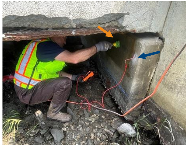
Figure 3. HCP testing of bent cap 4, showing reference electrode (orange arrow) and connection to reinforcing steel (blue arrow.)
